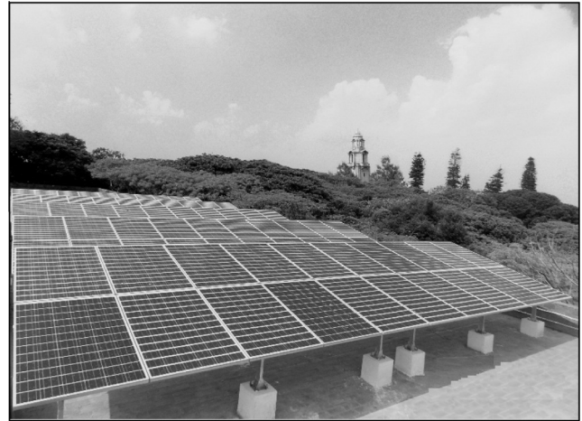
Fig. 1. Ariel view of the 20 kW p grid-interactive SPV system.
