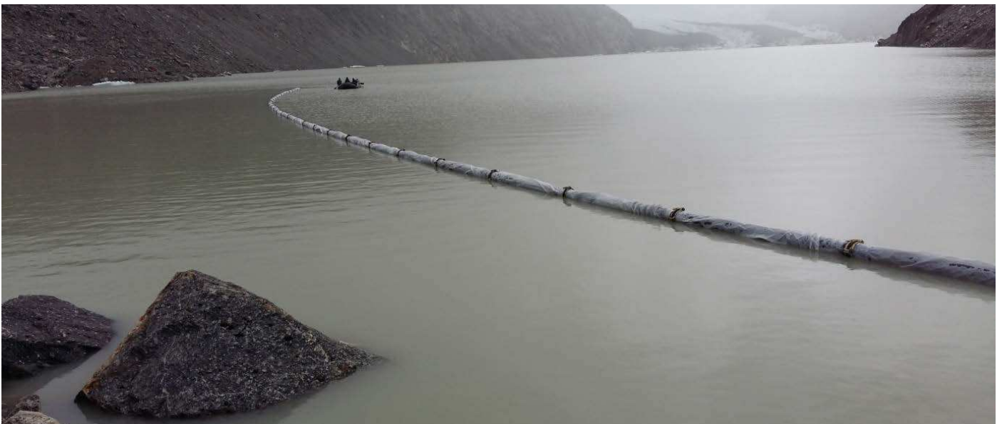
Siphon System after installation
